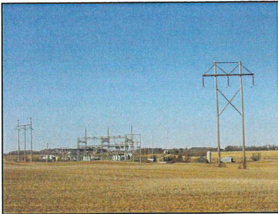
Figure 1 A Variety of Substations in Different Settings
